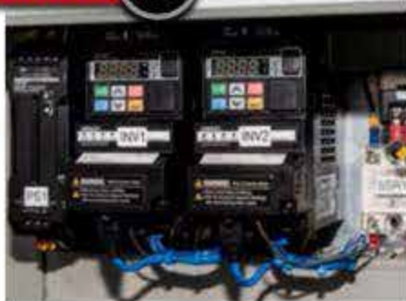
Omron parts include an S8VK Power Supply and MX2 Inverters.
